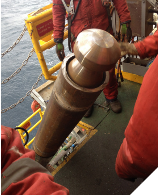
The embedded pawnheads enable quick abandonment and recovery or laydown, optimizing the allowable weather window for installation.
